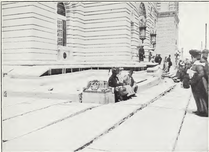
A. CRACKS IN MASONRY AND SETTLING OF OUTER TERRACE, POST-OFFICE BUILDING, SAN FRANCISCO.
